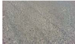
Figure 3: Rough Asphalt Road
