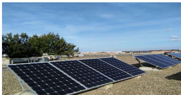
Figure 1: The PV plant installed on the roof
