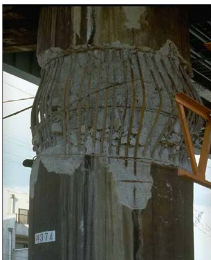
Figure.2: Failure Of Column Due To Lateral Buckling Of Longitudinal Reinforcement
